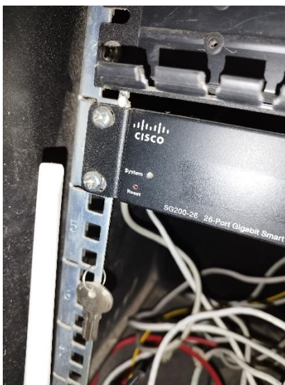
Figura 18. Cabina y Router Cisco SG200-26
